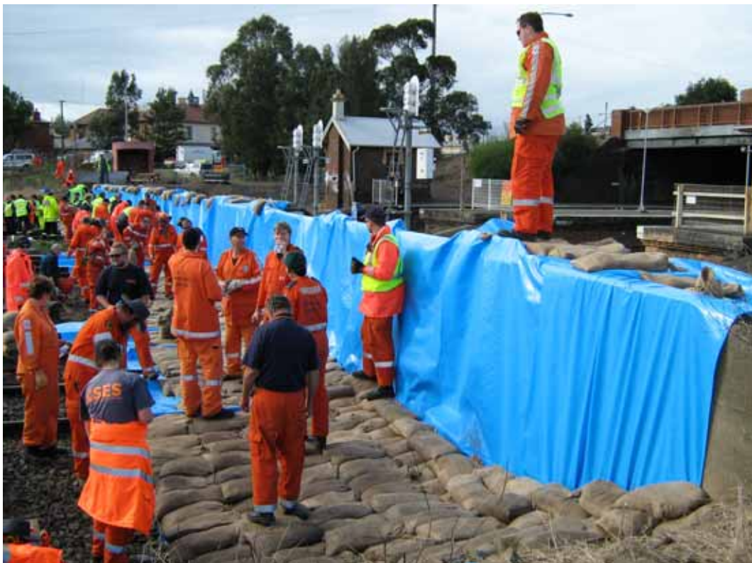
ACT & NSW SES teams work to seal the flood gates at the Maitland railway station. Photo: Rebecca Noble.
